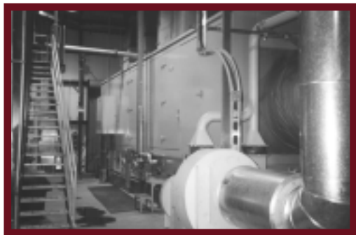
New Cogeneration Facility recently completed by ESI.
