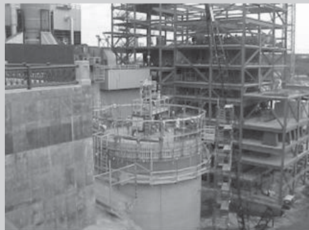
The heating plant is nestled on a 2-acre site in the heart of downtown St. Paul.
