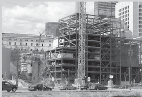
Due to site space, a large tower crane which was supported by concrete caissons and tied into the building steel was used to erect the unit.
